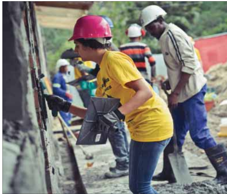
Builder Bob: Postgraduate student Salma Kagee slaps plaster on bricks. Kagee was one of the Faculty of Commerce’s volunteers helping to extend the Philippi Children’s Centre. It’s linked to the R150 million Starting Chance Campaign, initiated by the Southern Africa Sustainable Development Initiative.
