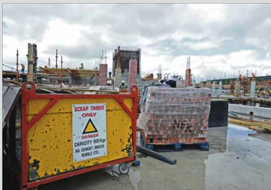
Be warned: Construction sites are dangerous. Safety signs are there to protect you.
