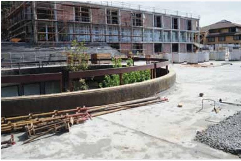
Brick by brick: The new Student Administration Building going up on middle campus.
